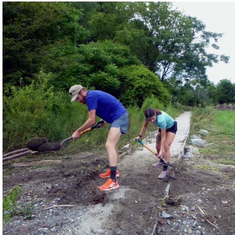
In Richmond, the Johnnie Brook boardwalk was buried but unbroken.
