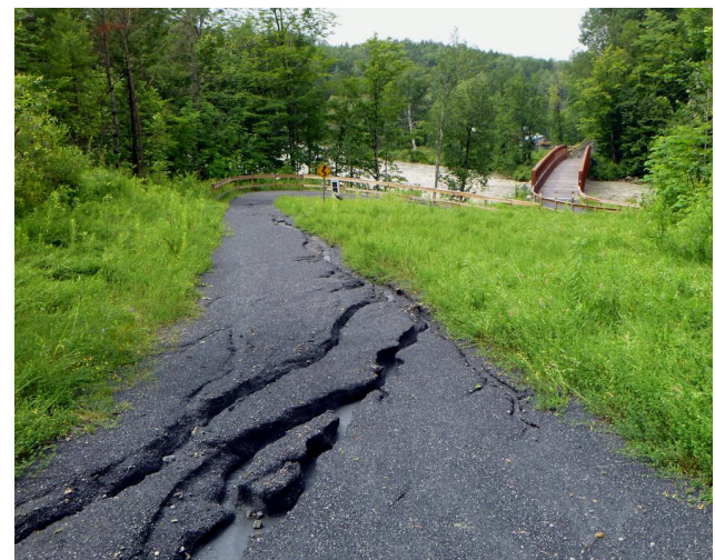
Major structures like the Winooski Bridge did well in the big storm, but there were uncountable smaller washouts to repair. After finishing all that this Fall, we are ready to resume progress on new trail construction in East Montpelier next Spring.
