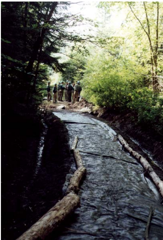
Use of Geotextile on a wet section of the Cross Vermont Trail in Newbury Credit: Eric Scharnberg
